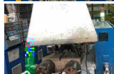
Exhaust gas treatment device in a workshop
